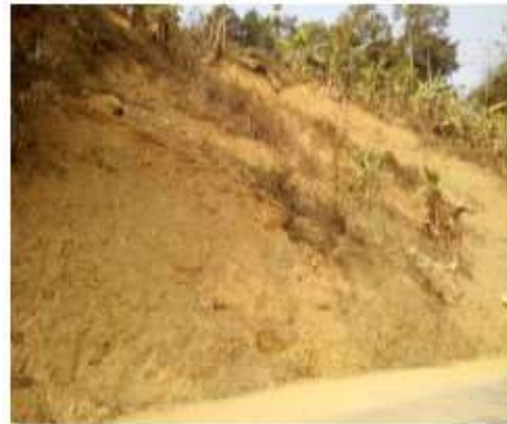
Landslide location code: L-4
