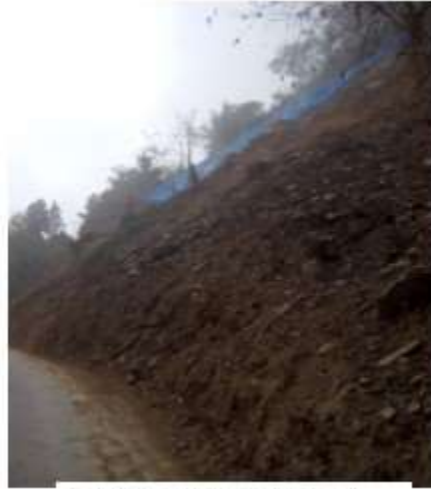
Landslide location code:L-12
