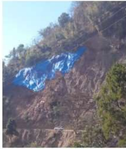
Landslide location code: L-6
