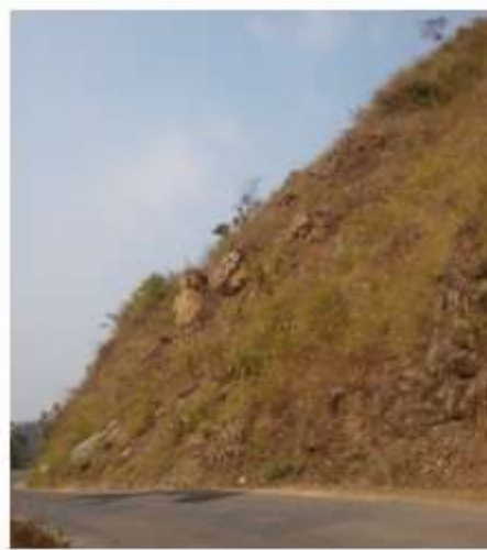
Landslide location code: L-11
